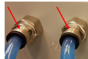
Figure 10-10 Chiller's Water Tubes
