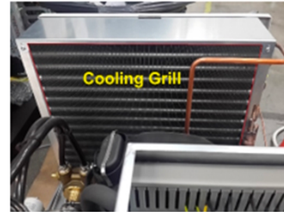
Figure 10-11 Chiller Cooling Grill
