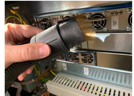
Figure 9-12 Vacuum Cooling Fans
