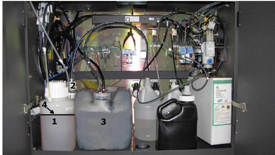
Figure 2-4: Waste container cabinet
