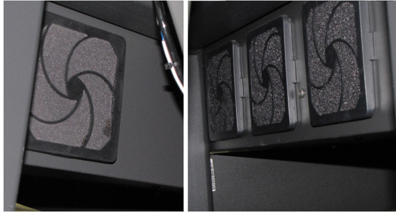
Figure 2-48: Cabinet air filters - ink cabinet (L) and computer cabinet (R)
