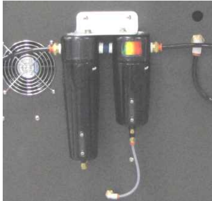
Figure 2-40: Nitrogen system filters
