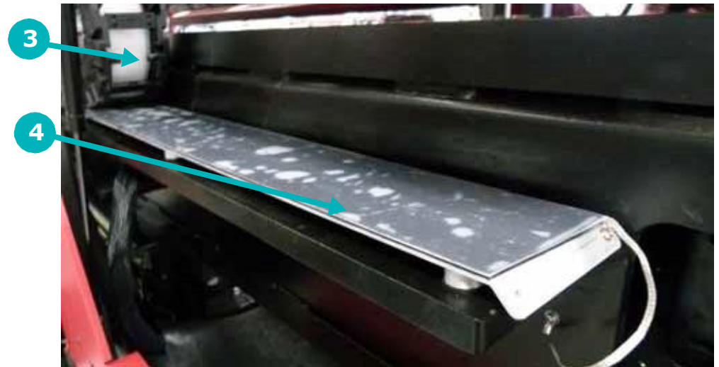
Figure 2-39: Cable carrier and shelf
