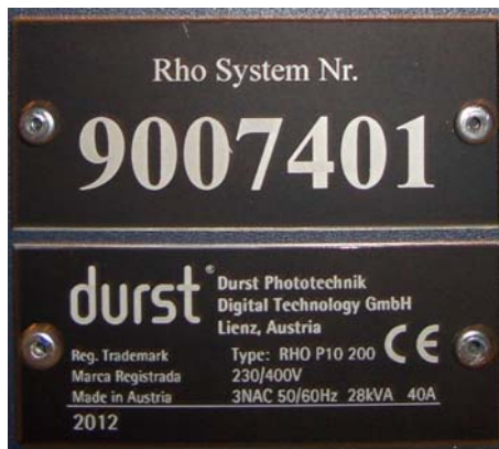
Fig. 2 Rating plate (location 13: door at main switch)
