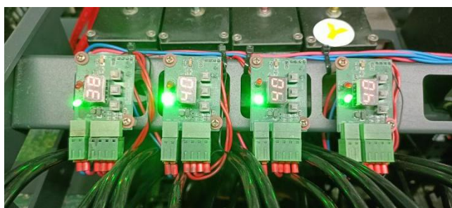
Fig. 127 Operating state of temperature control board
