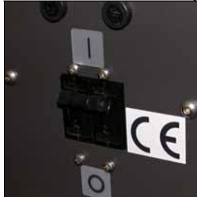
Figure 7: Main AC Breaker – On position
