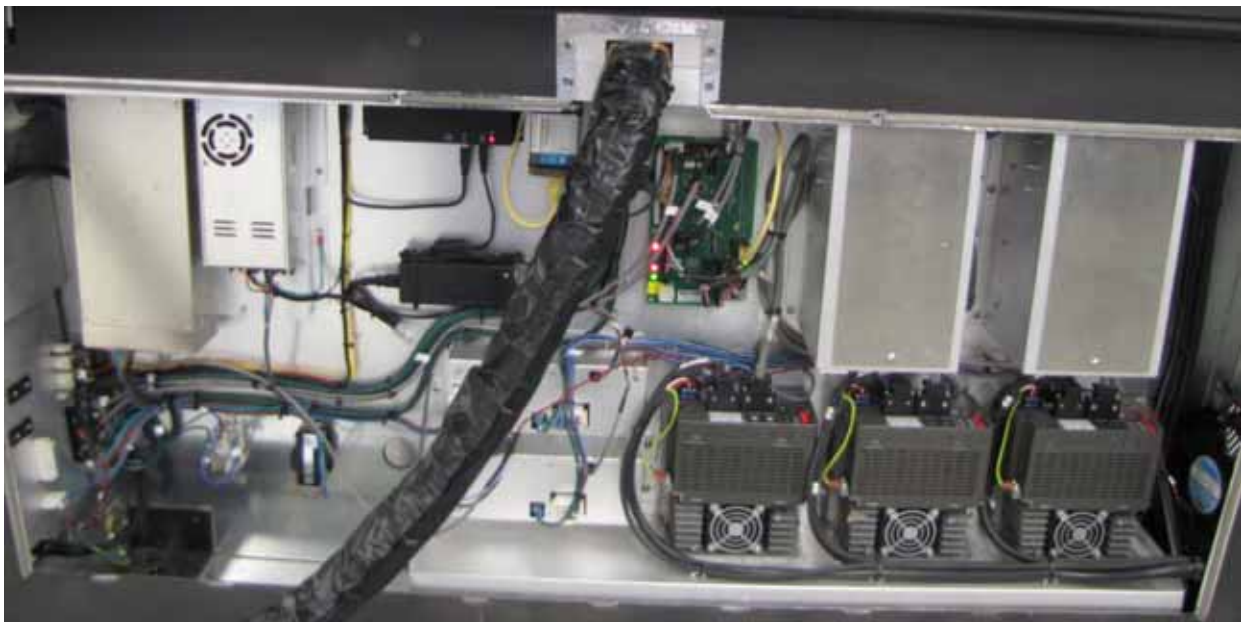
Figure 1-13: Printer Electronics Cabinet
