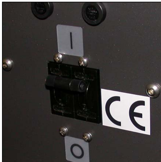
Figure 4: Main AC Breaker - On position
