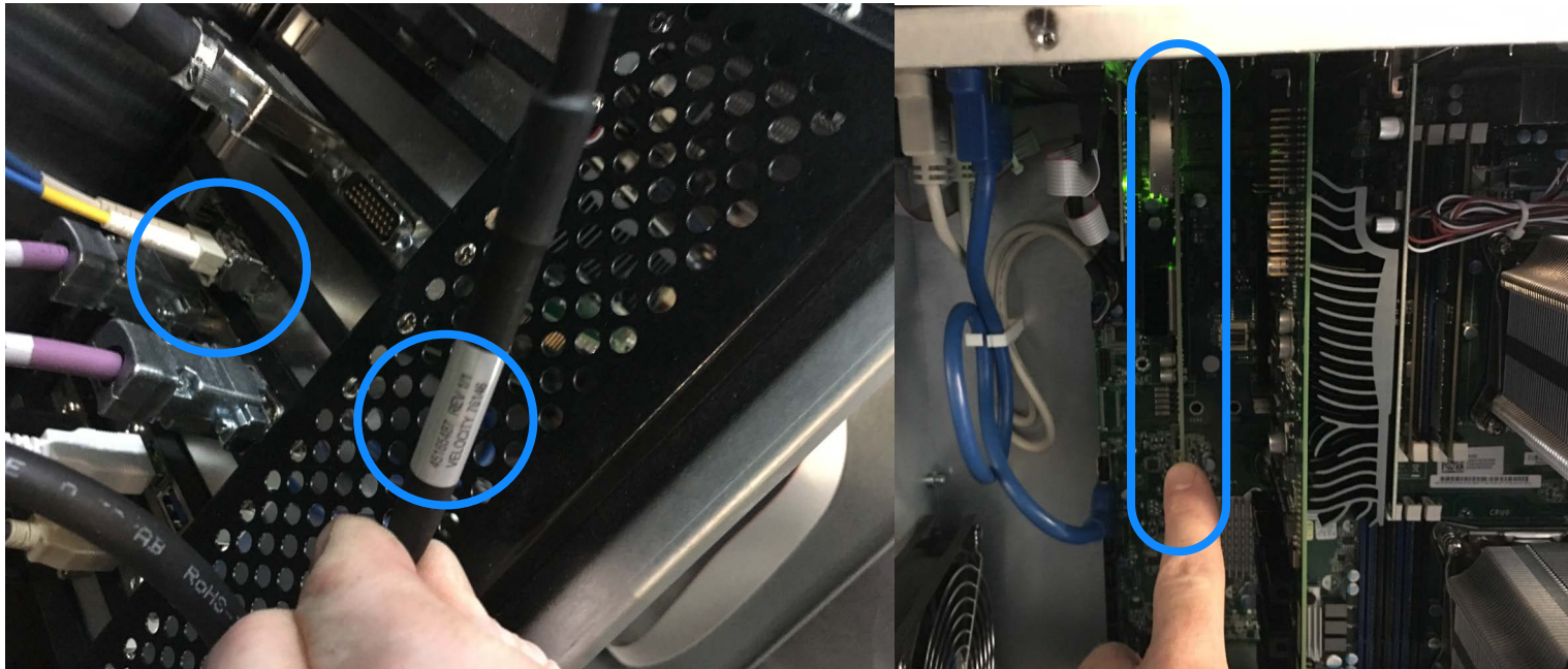
Figure 1-9: Ferrari Fiber Optic Cable, Left, and Ferrari Light Board, Right
